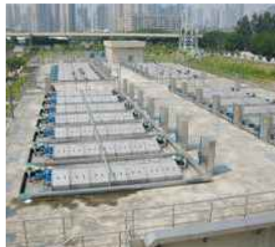
24 installed HUBER Disc Filter RoDisc® units.
